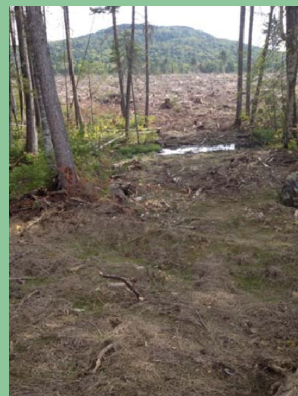
The Company’s guidelines for installing and removing temporary crossings were found to be effectively implemented to reduce the operational impacts to streams. This picture also shows how natural drainage is being maintained and sediment control measures implemented following the removal of a crossing.
