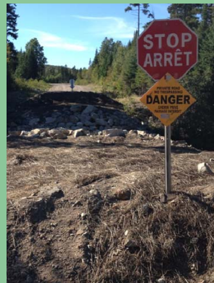
The field audit observed a number of examples of well implemented road and bridge deactivation (above) and road construction and bridge installation (at left) practices.
